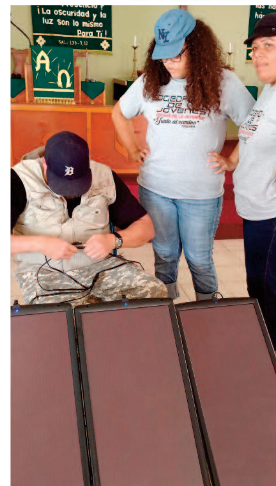
Above: Here he is pictured assembling one of many units in the hardest hit area on the south east side of the island.
